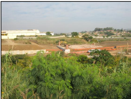
Figure 7: Photograph of the current construction activities adjacent to the northern boundary of the site.
