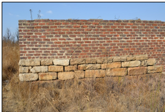
Figure 3. Exterior wall of the garage indicating the various building materials that were used for construction (Photograph: M. Naude 2013).
