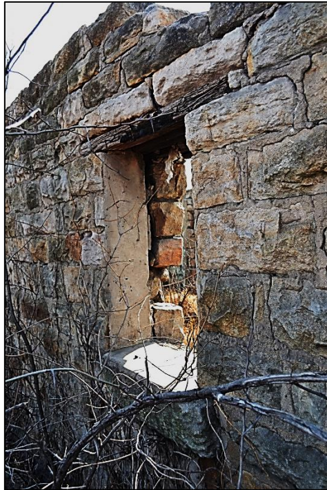
Figure 9. Sandstone window sill and timber lintel (Photograph: M. Naude 2103)
