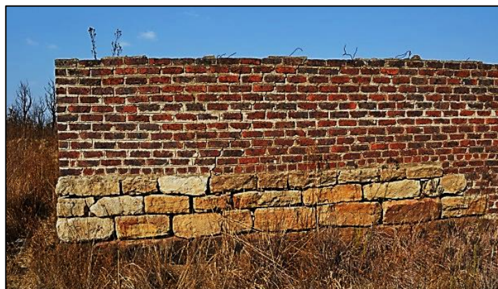
Figure 12. Original sandstone base that could have served as a wall or may have been built specifically as base for the garage wall (Photograph: M. Naude 2013)
