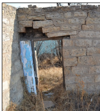
Figure 18. Disintegration of the walling due to permanent exposure to rain and sun resulting in the destruction of the entire building (Photograph: M. Naude, 2013)
