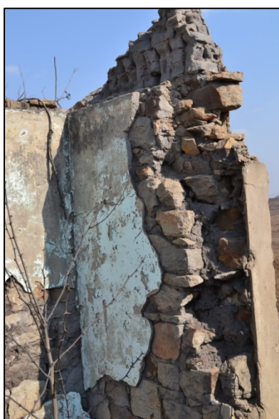
Figure 7. Remnants of the front gable seen from the interior (Photograph: M. Naude 2013)
