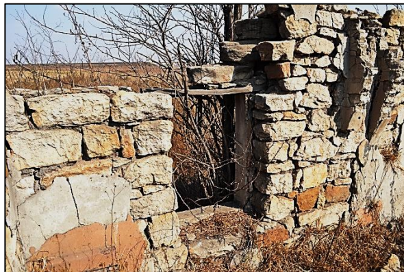
Figure 10. Remains of timber lintel of window (Photograph: M. Naude 2013)
