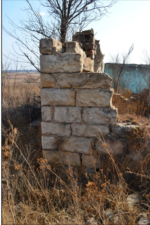
Figure 8. Quoining at the one corner of the dwelling that has remained intact demonstrating the level the stone was dressed (Photograph: M. Naude 2013)
