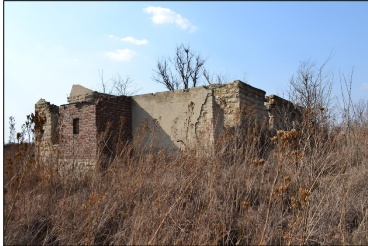
Figure 1. Exterior of the dwelling indicating the degradation of the building (Photograph: M. Naude 2013)
