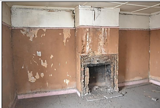
Figure 5. Remains of clay plastering in the principal lounge. The mantelpiece has been removed.
