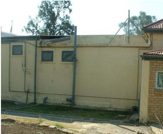
Gutters falling down
