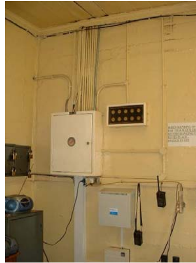
All surface mounted electrical installation
