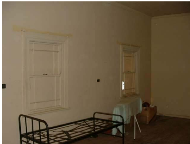
Non-assignable room with mixed usages such as ironing, redundant storage etc. Note the painted windows and the open space within the room which is symptomatic of poor space planning.
