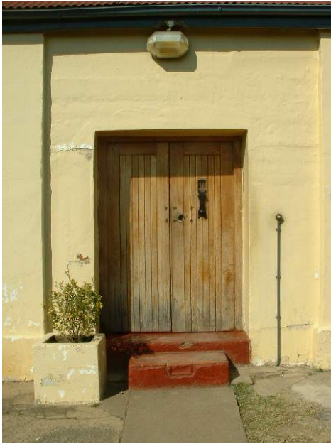
Poor condition of front door
