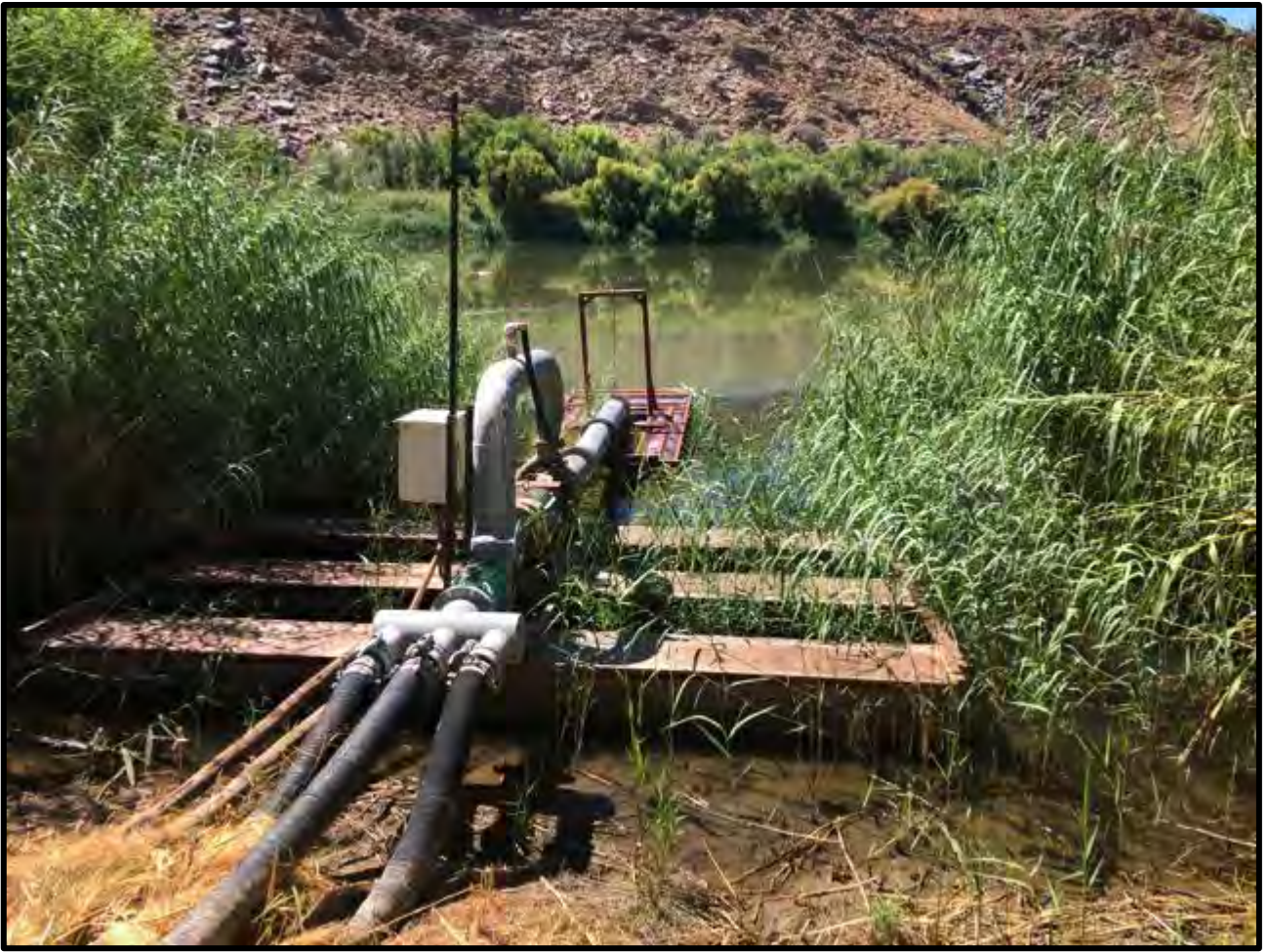
River pump station
