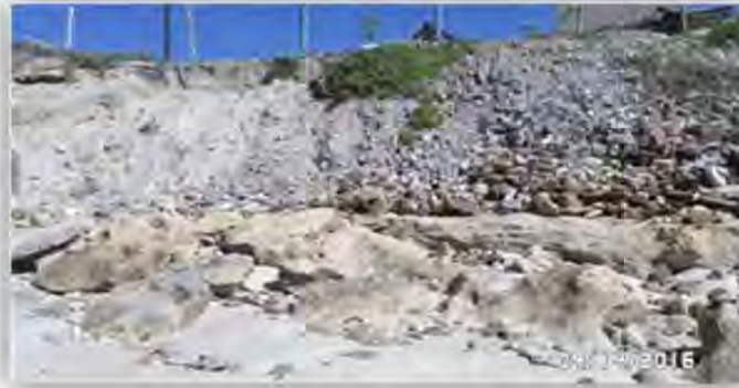
Figure 2: Eroding harbour embankment
