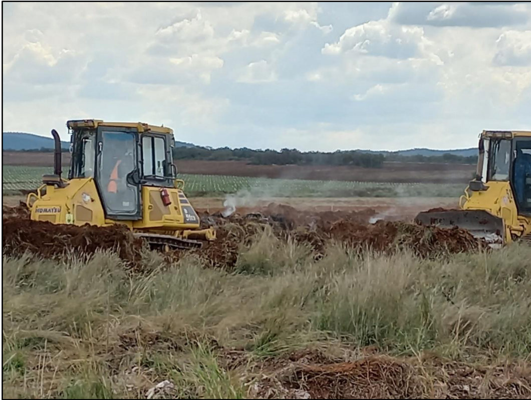
Figure 4: Heavy machinery at work preparing the site for orchard landscaping. The smoke in the background is from burning piles of removed vegetation.
