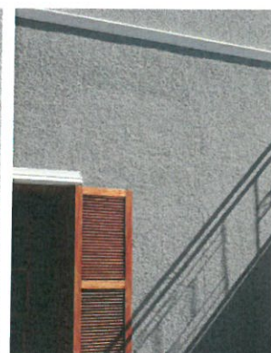
Evidence of old doorway
