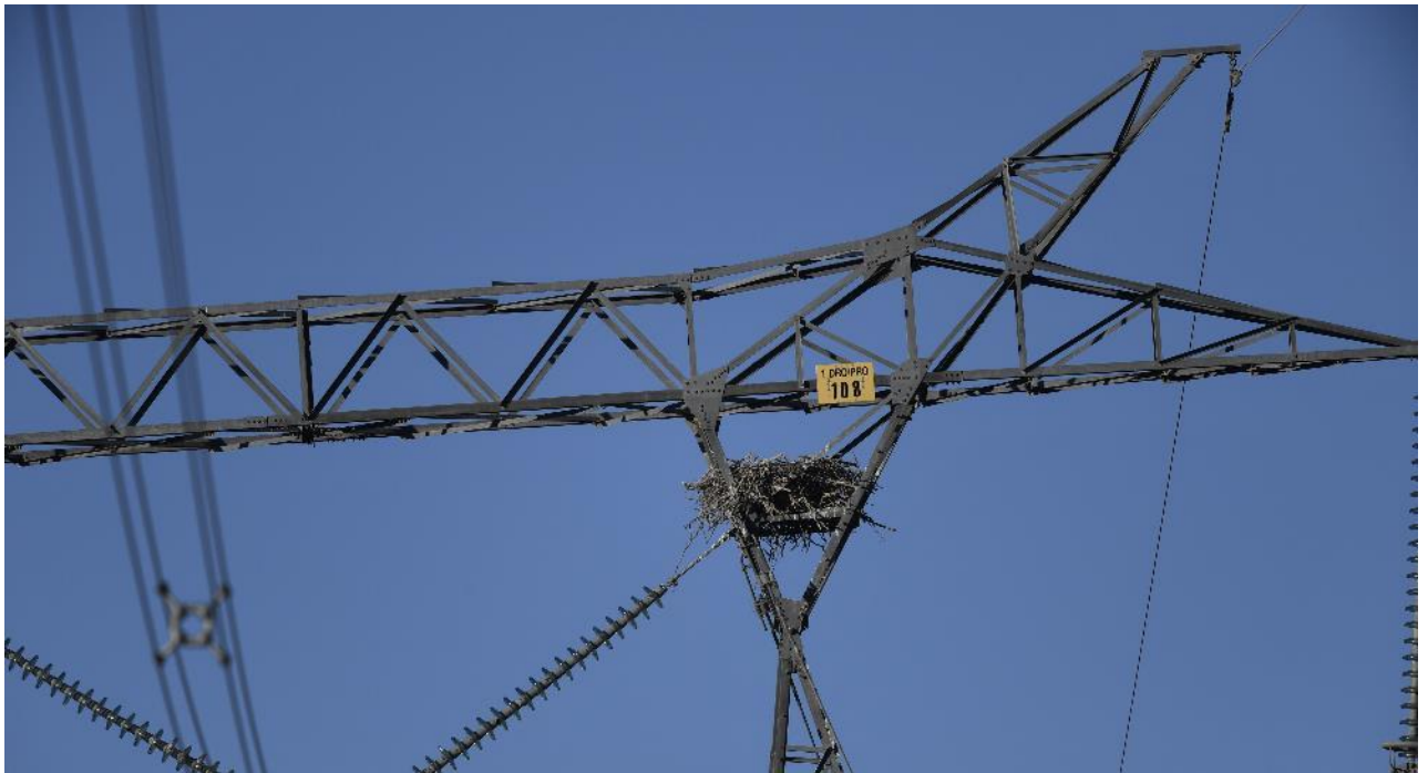
Figure 2: Tower 108 of the Droërivier-Proteus 1400kV transmission line, where the Martial Eagle nest is present, located to the west of the application site.
