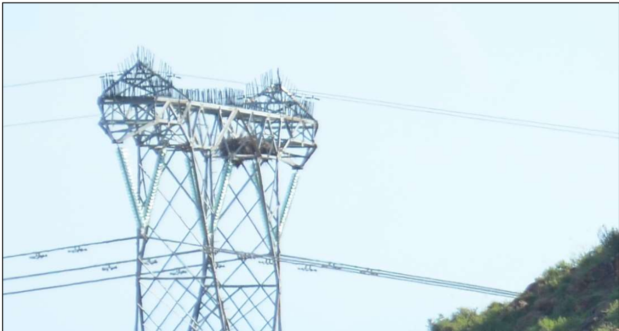
Figure 9. A close up of the Verreaux's Eagle nest constructed within the trellis structure of the pylon.
