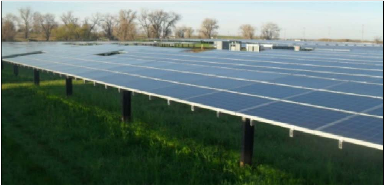
Figure 7: Frontal views of the PV arrays mounted on horizontal 1-axis tracker
