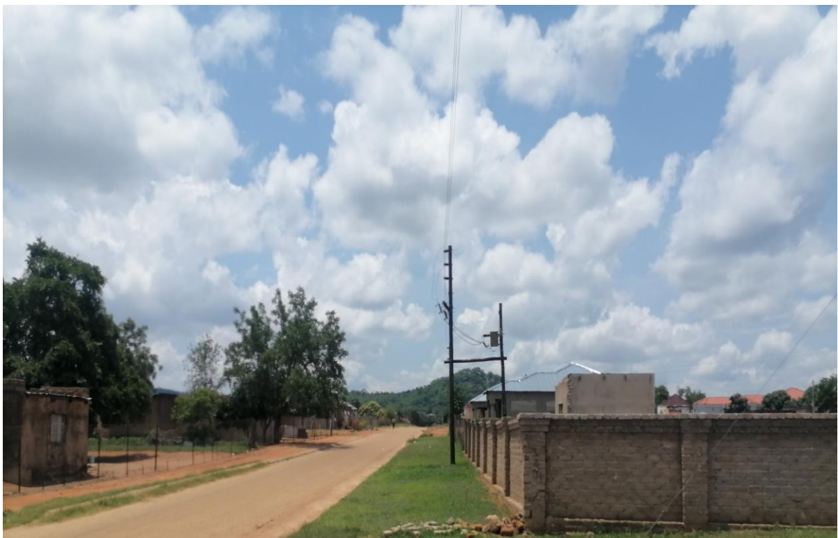
Photo 2: Shows the existing powerline on site
