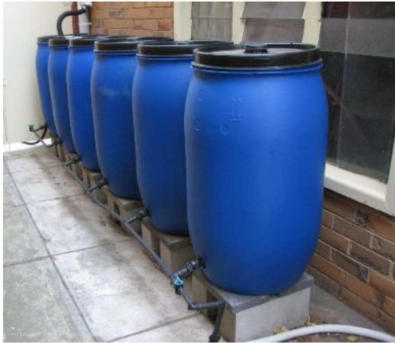
Figure 4: Typical example of water storage tanks
