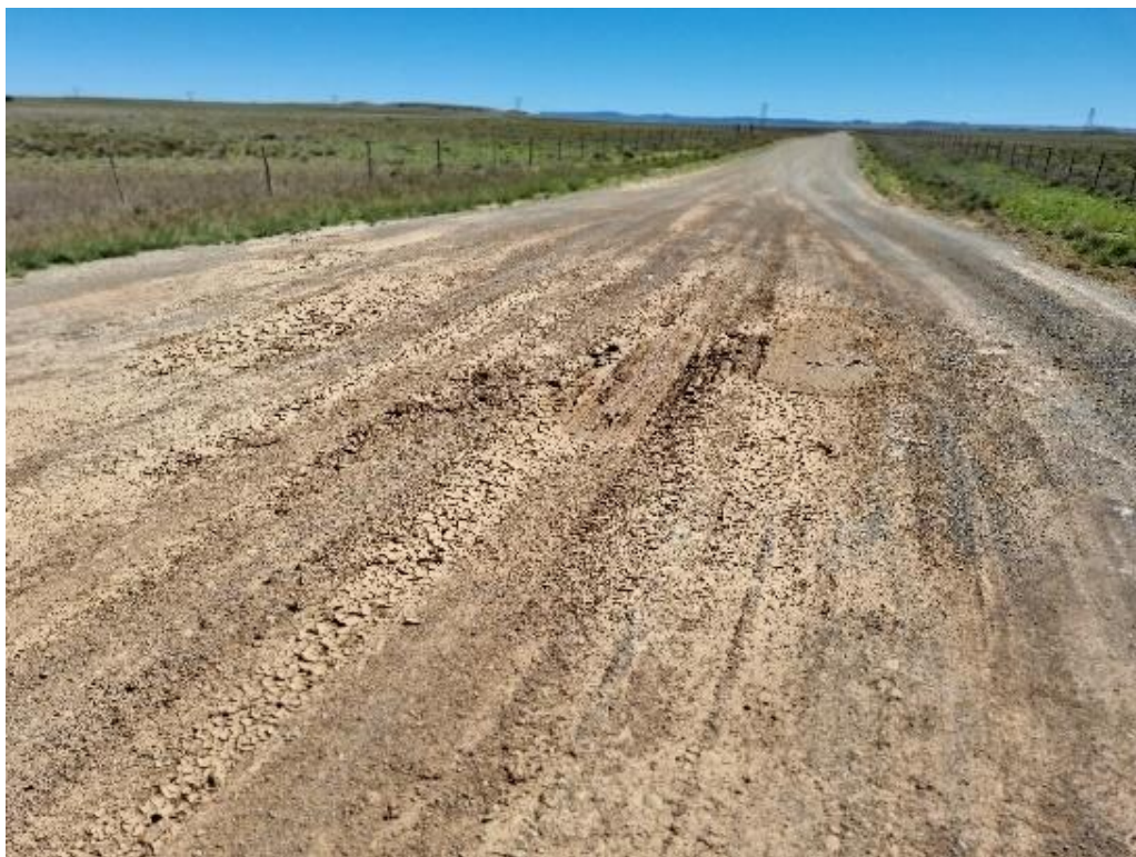
Photo 3: Possible seep (and associated road failure) adjacent to the servitude of the public 'Burgerville' District Road (facing Northeast).
