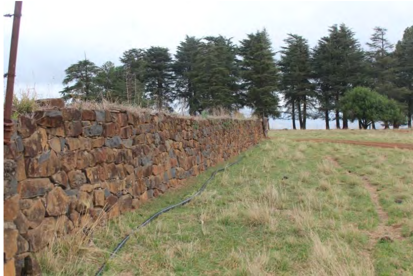
Figure 6: Manmade rupicolous habitat just east of the Manure Processing Plant. Note the exotic kikuyu grass and pine trees in the photograph.
