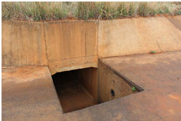
Figure 10: A drainage line underneath the water canal west of the study site of Pig House 3.
