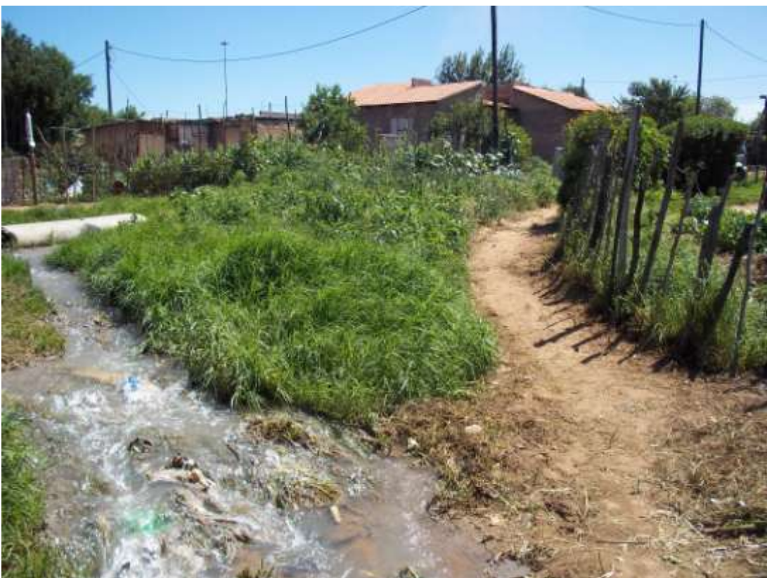
Photo 6: South-western perspective of the sewer connector line.
