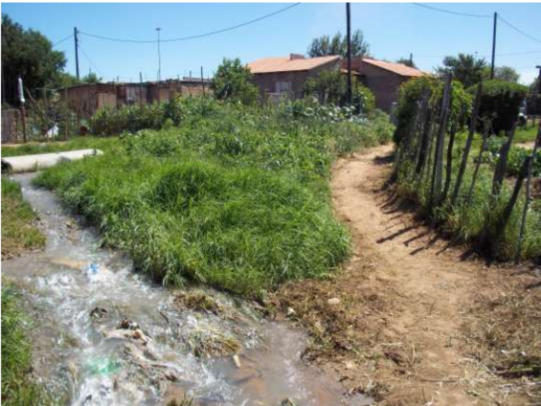
Photo 6: South-western perspective of the sewer connector line.
