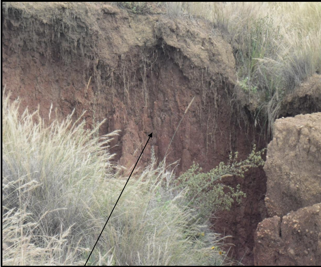
Photo 2: showing eroded banks along the existing track.
