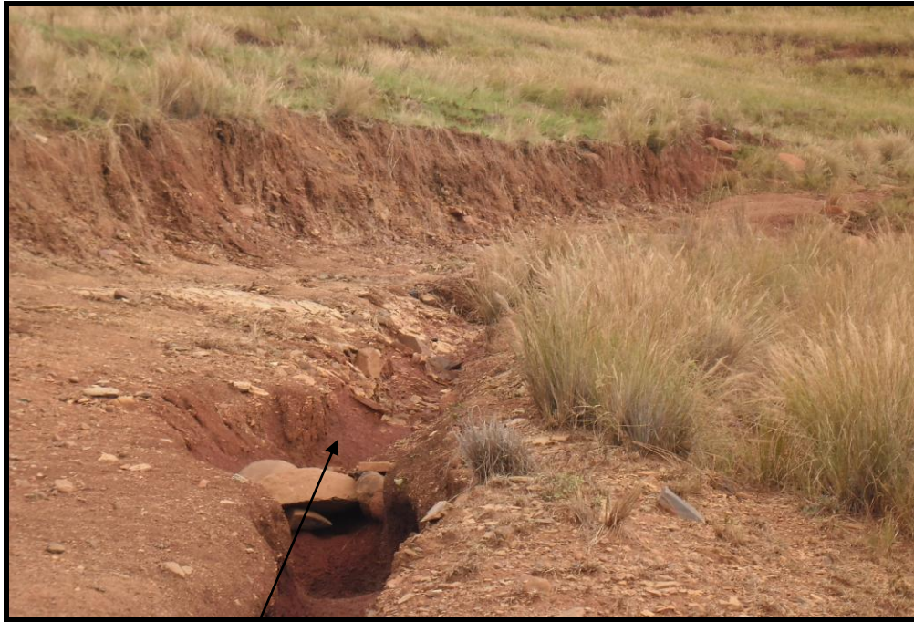
Photo 2: showing gully erosion as a result of poor drainage of the existing road
