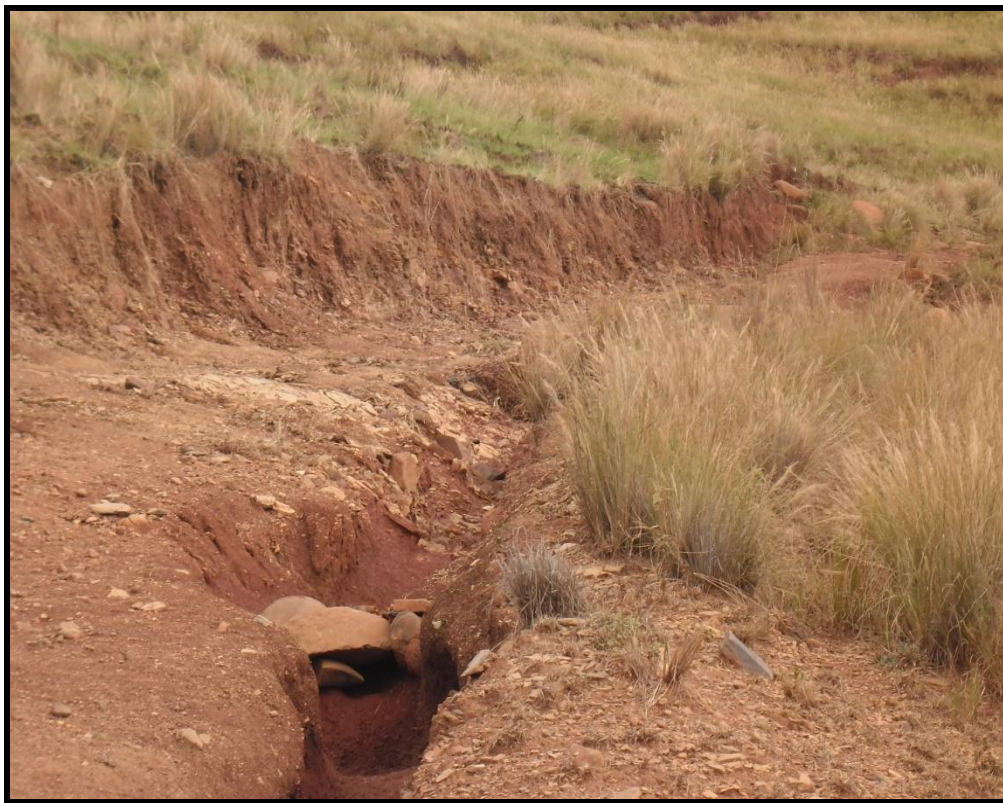
Photo 1: showing gully erosion as a result of poor drainage of the existing road.
