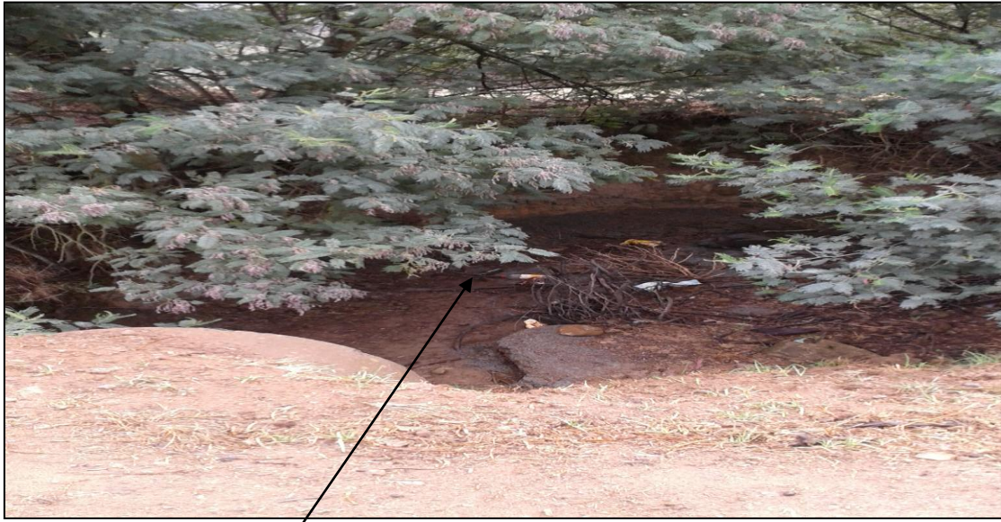
Photo 2: showing erosion as a result of poor drainage of the existing track
