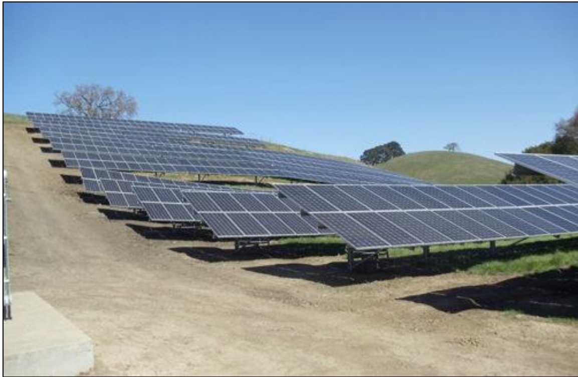
Figure 5: Image showing an example of a ground-mounted solar array ascending up a hill. (Source: RBI Solar, www.solarpowerworldonline.com )
