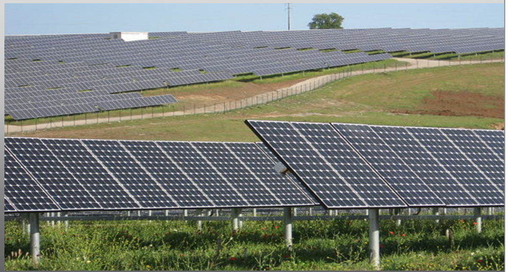
Figure 1: Illustration of photovoltaic (PV) arrays on a solar power plant.
