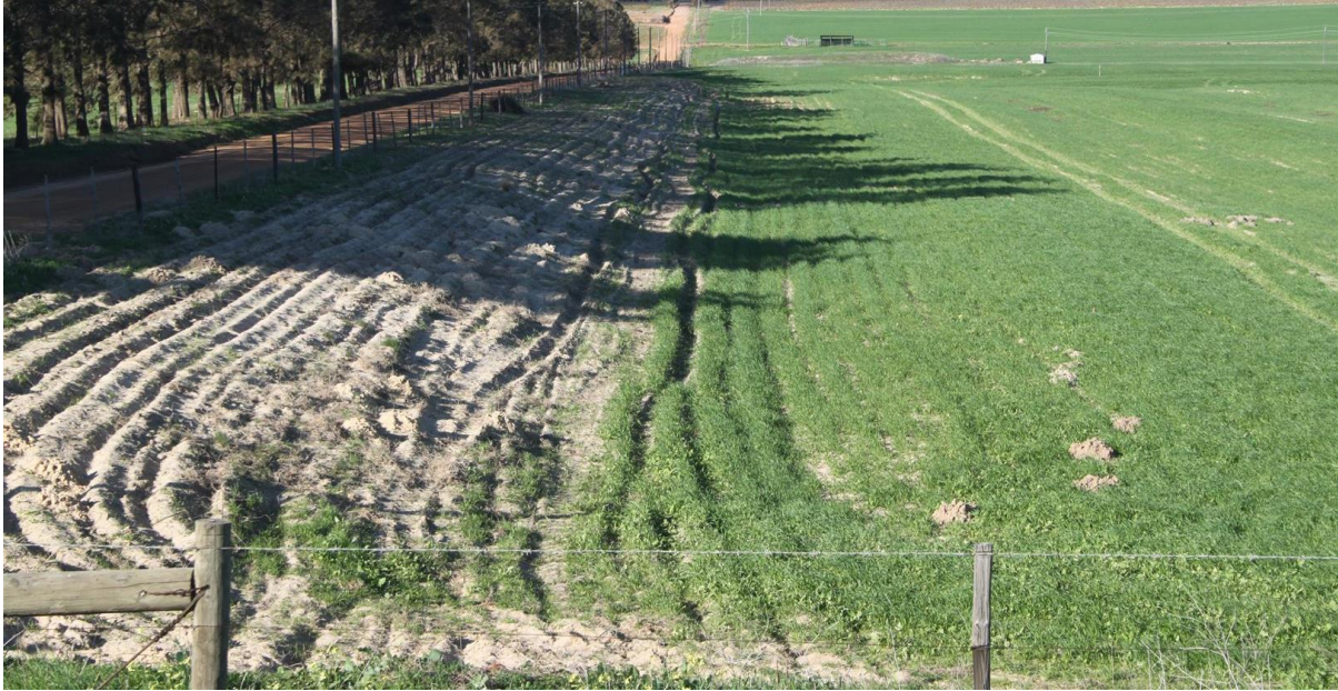
Photo 2: Typical Borrow Pit rehabilitation with full topsoil replacement and revegetation by pasture seeding on the floor of the excavation, and scarification of 1:3 side slope ready for hand seeding.
