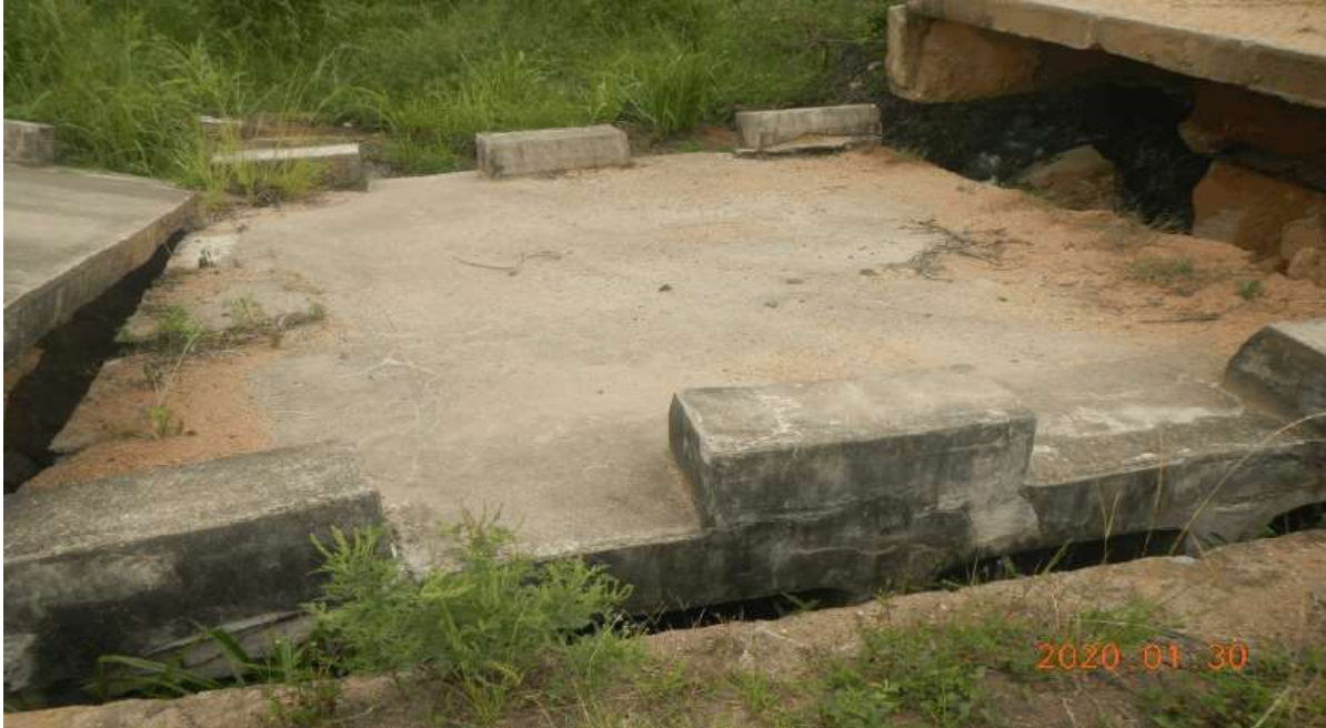
Existing bridge in vertical collapse
