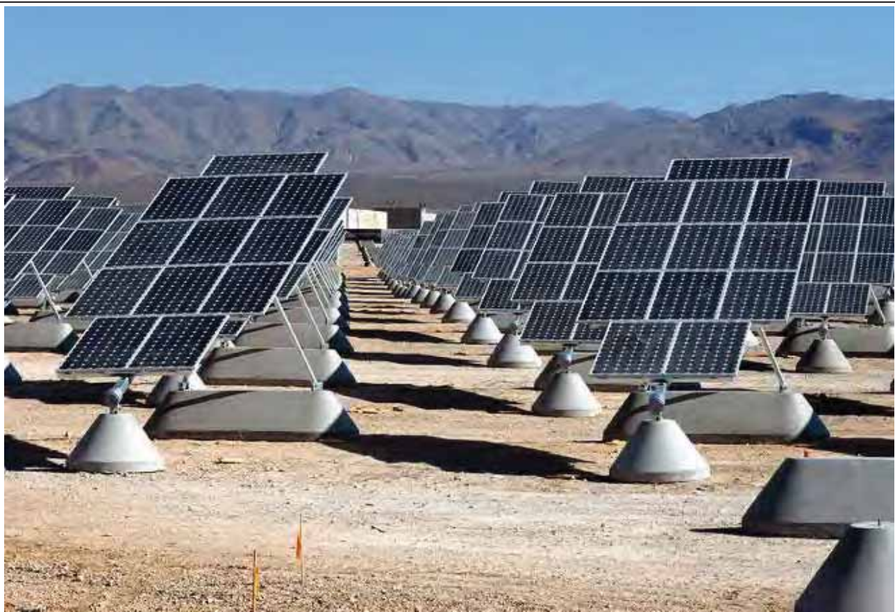
Figure 2: Tracking PV array
