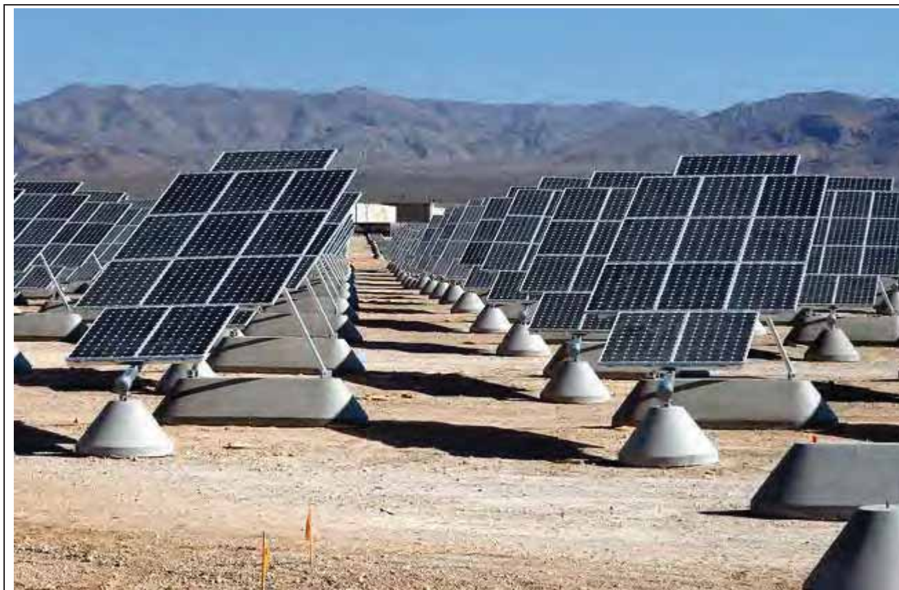
Figure 3-2: Tracking PV array
