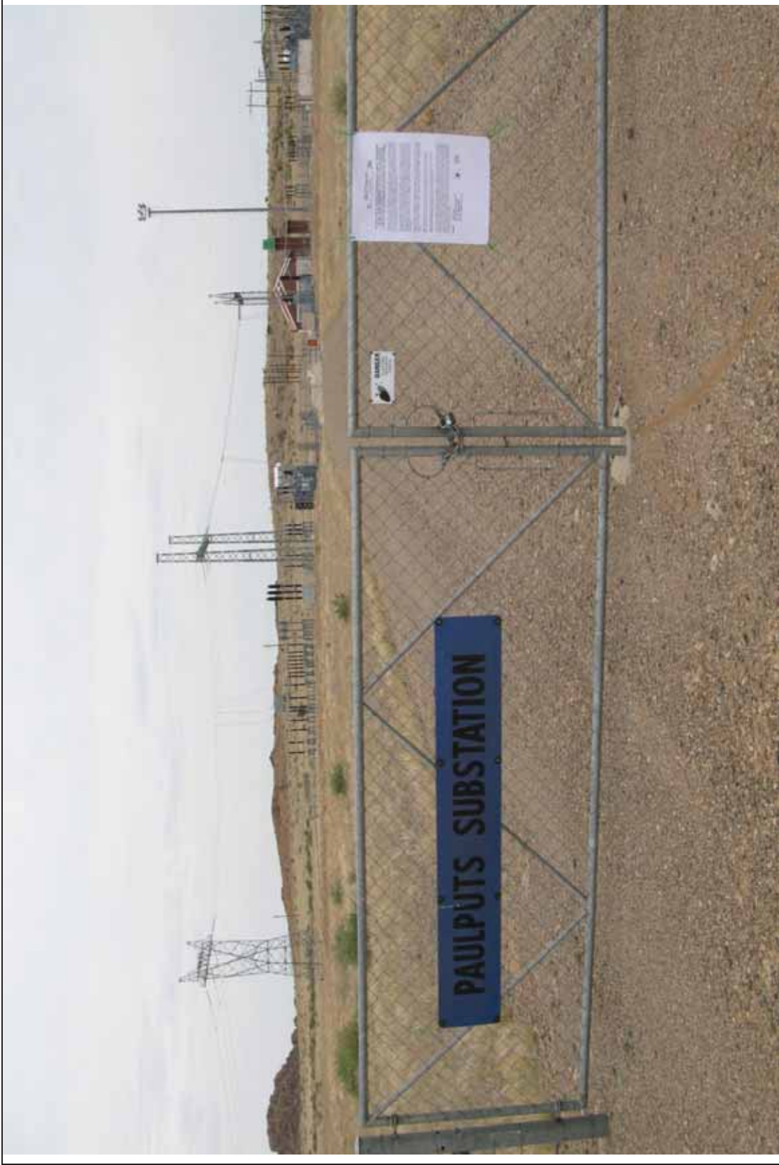
Site notice on Konkoonies site boundary fence Paulputs substation
