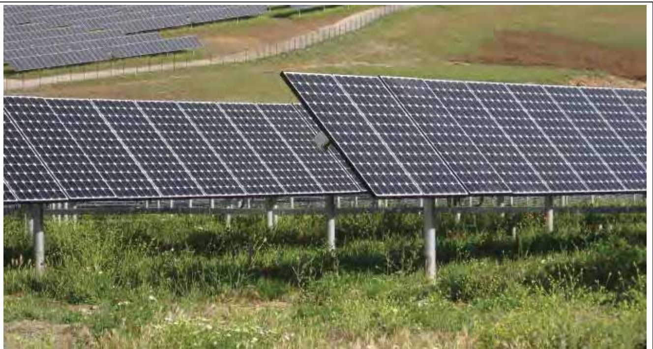
Figure 1: Fixed tilt PV array
