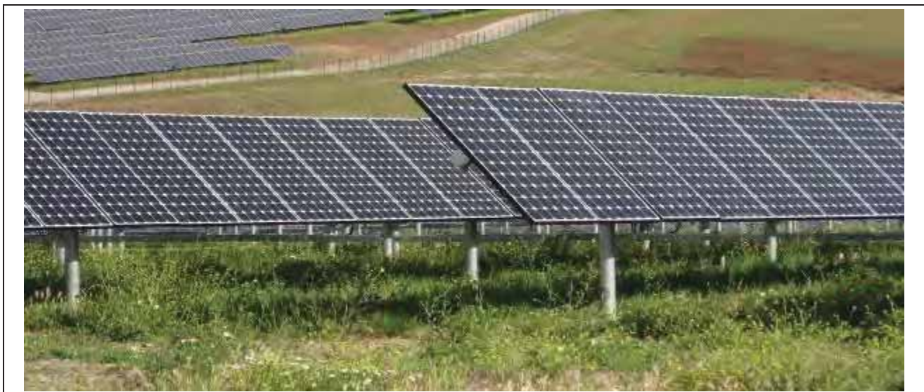
Figure 3-1: Fixed tilt PV array
