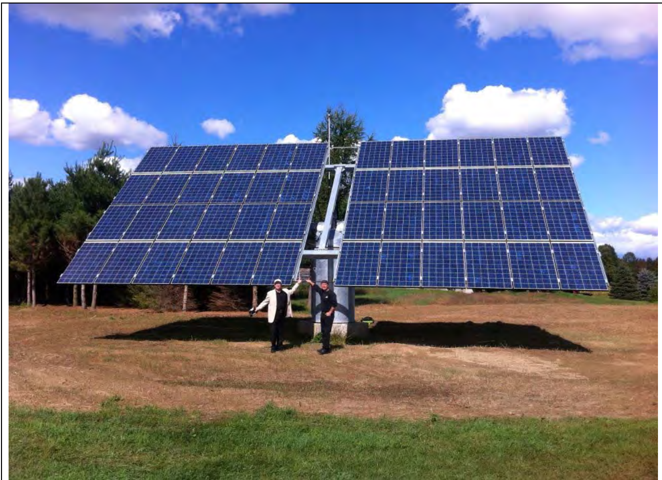
Figure 3-2: Tracking PV array (sourced http://solarblog.ca )
