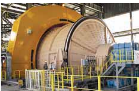
A typical zinc concentrator plant
