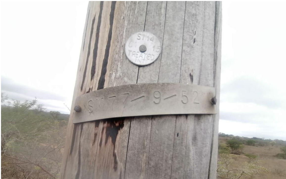
Photo 1: Shows the existing pole number on site
