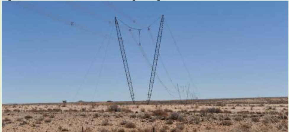
Figure 6: The Aries – Kokerboom 400kV high voltage line
