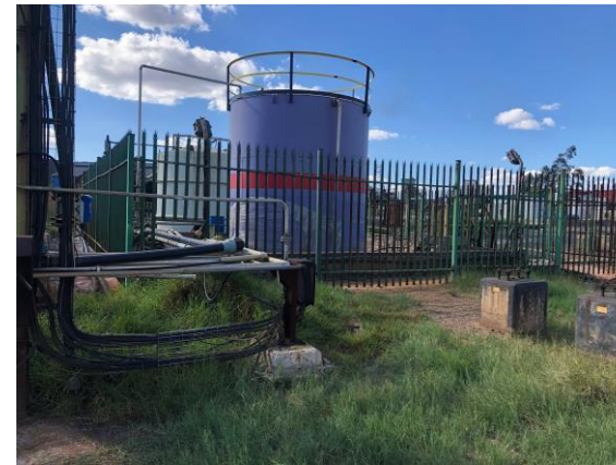
Existing structures associated with the Chemical Plant surrounding the area of the proposed location of the new tanks (north)
