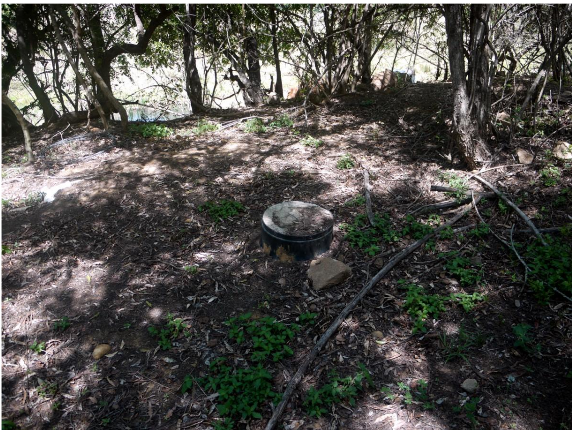
Plate 10, Rock Pools, septic tanks close to the edge of the water course.
