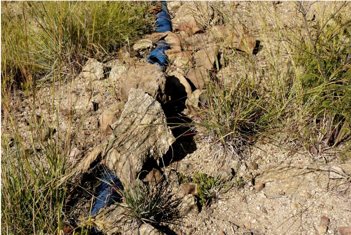
Plate 32, Leopard Rock, original pipe runs were laid on the surface and covered with rocks.
