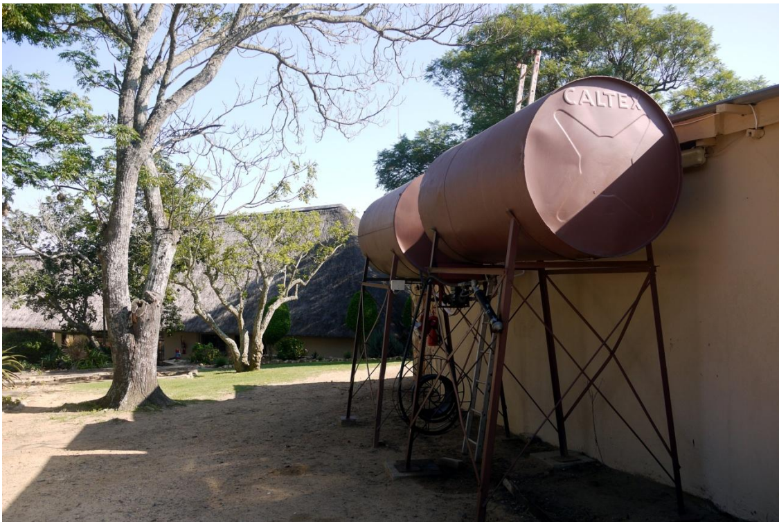
Plate 22, Existing fuel tanks at the farmstead. It is likely that a greater quantity of fuel and other hazardous materials will be required within the service area. Careful consideration of methods to minimise associated risks will be required. Fuel storage will require a bunded area.
