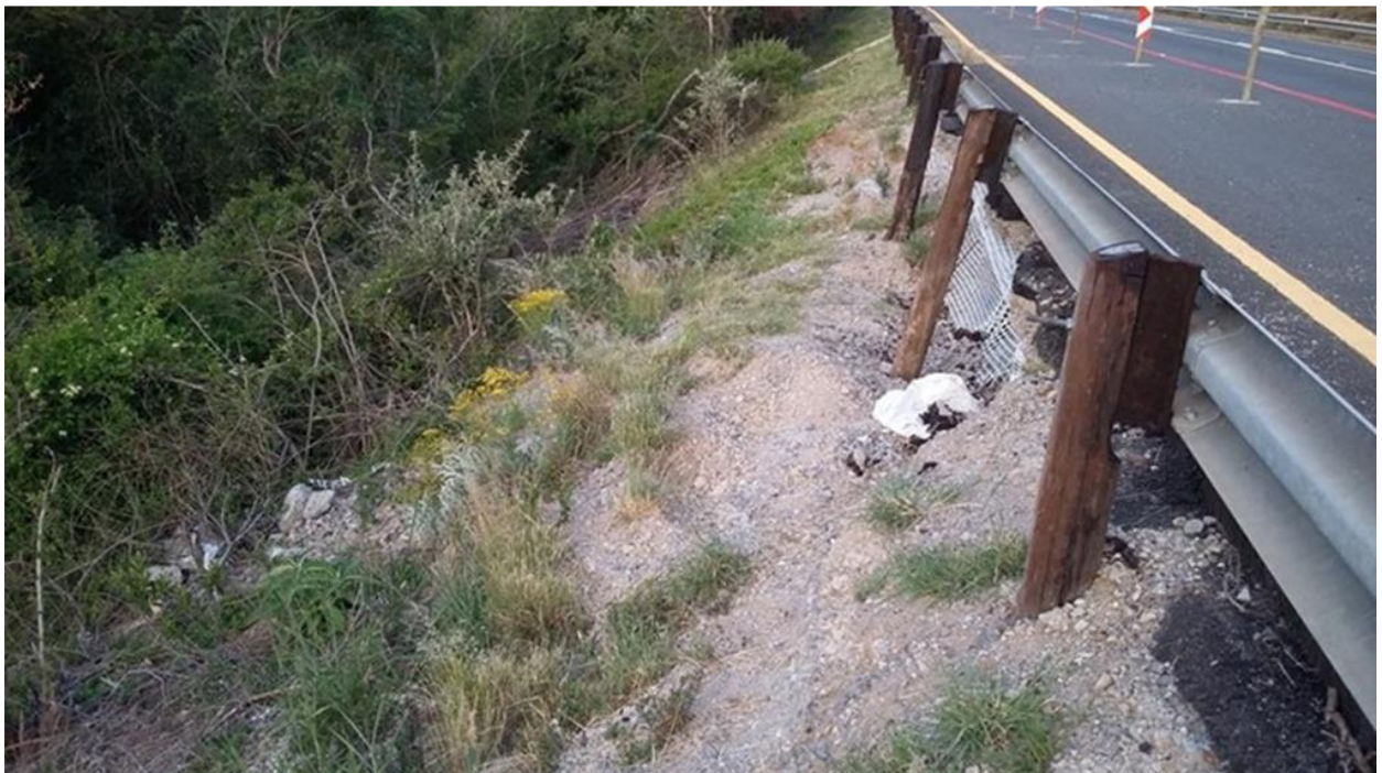
Figure 3: Gaps in the existing bitumen pre-mix curbs and resultant erosion and slumping down the embankment at approximate chainage km 43.130
