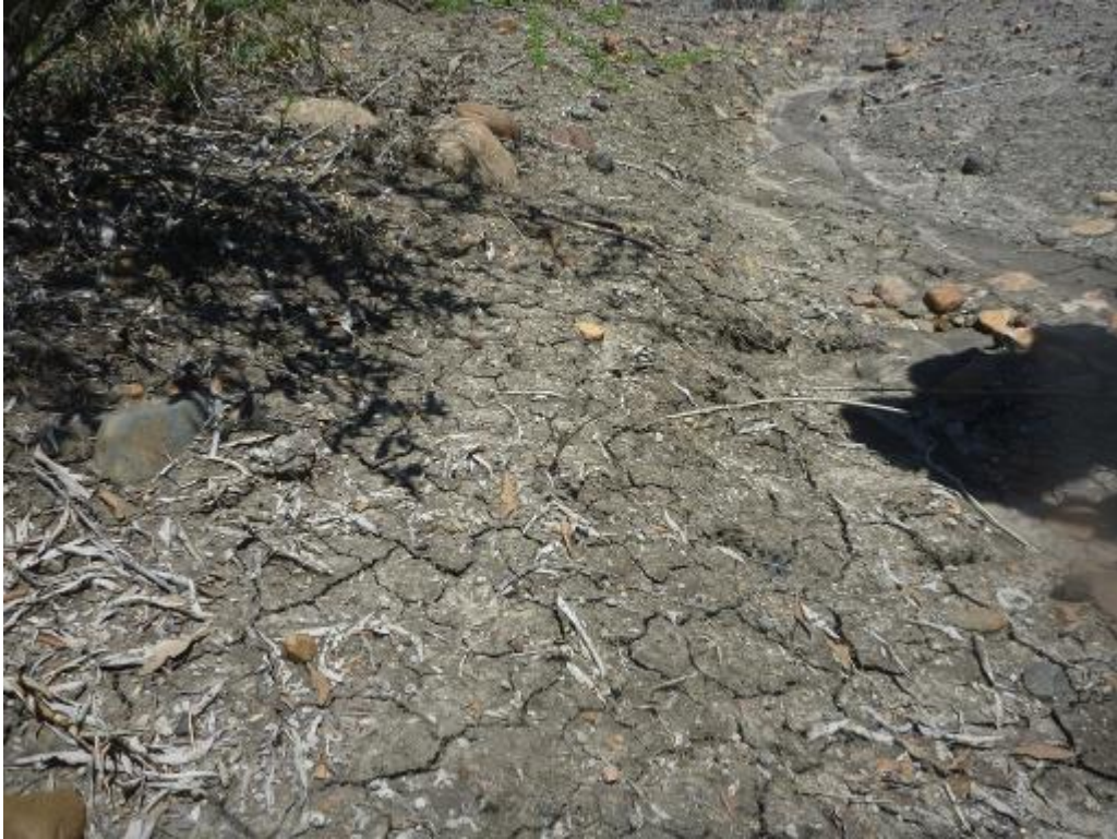
Figure 10 Swell-shrink potential is manifested typically by the formation of conspicuous vertical cracks in the dry state
