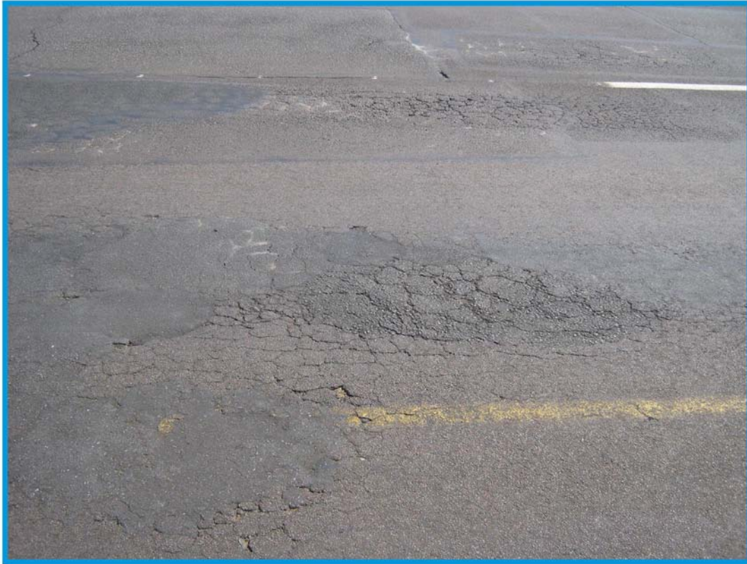
Photo 17: Patching on the R556 also Cracked with Signs of Pumping
