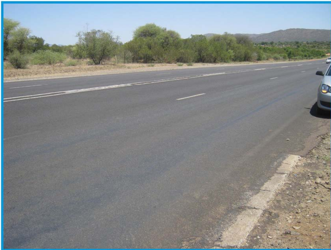
Photo 18: Minor Bleeding along the R565
