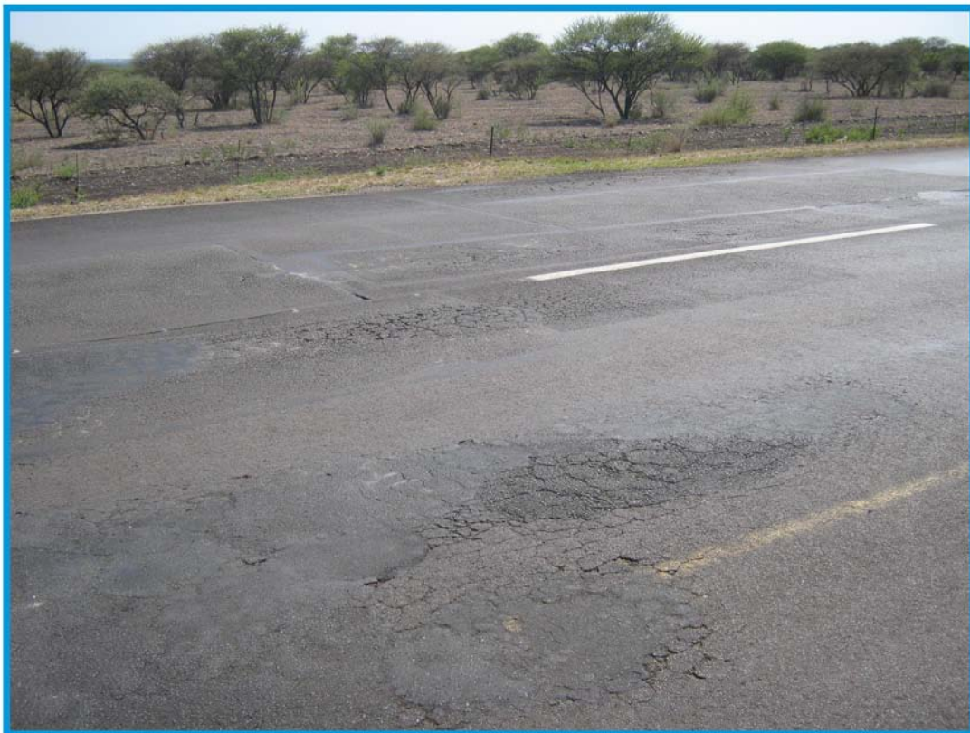
Photo 16: Crocodile Cracks, Patching and Bleeding on the R556
