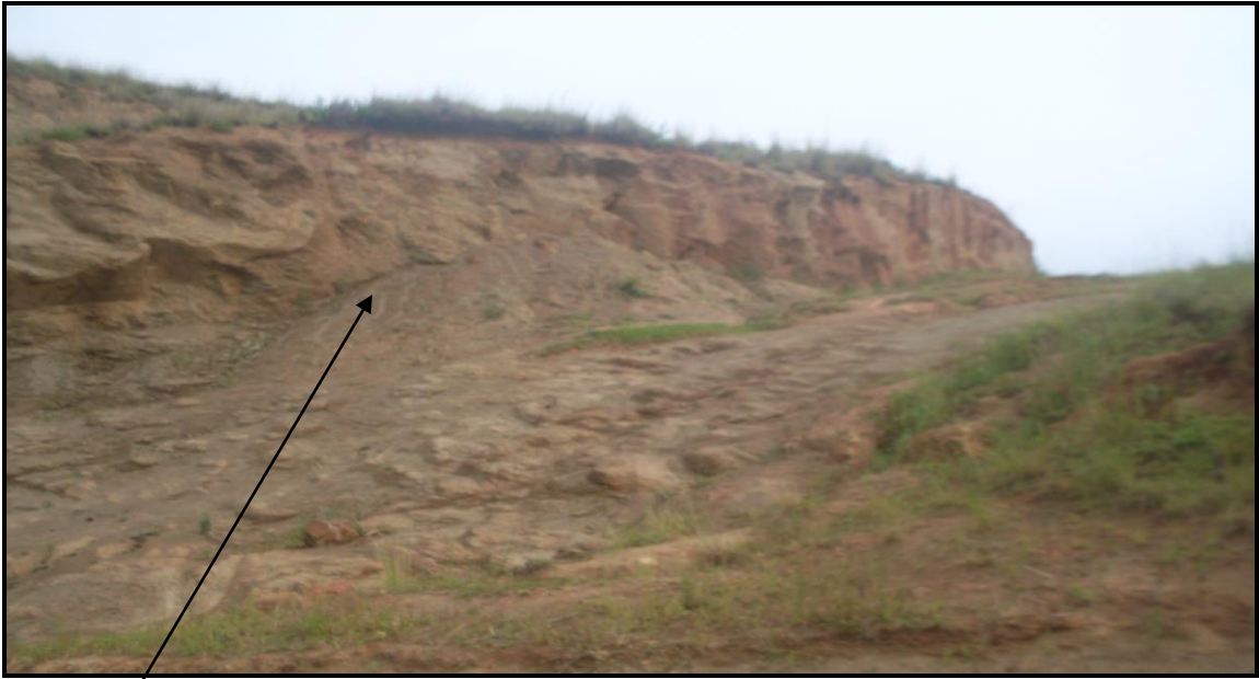
Photo 2: showing erosion as a result of poor drainage of the existing road
