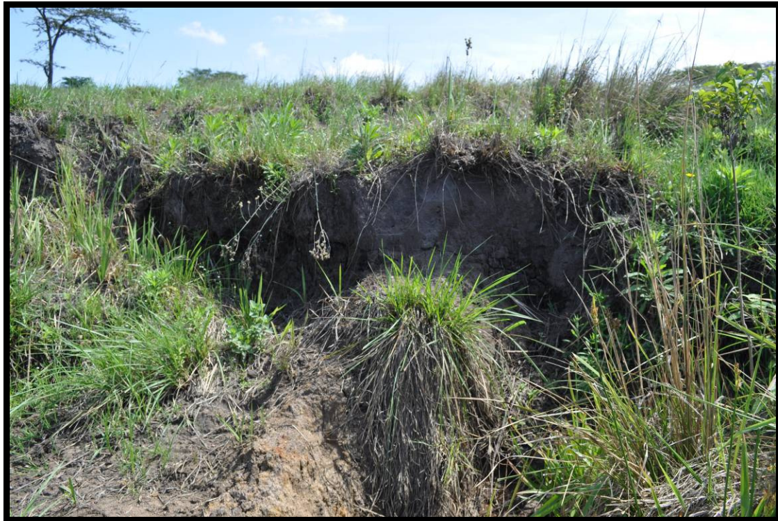
Figure17. A head cut erosion was observed within the southern seasonally inundated seepage wetland. Adequate gabions and gabion mattresses with sediment trapping geo-textiles should be installed to prevent further erosion up the seepage areas. The eroded area should be fenced off preventing further trampling and disturbances from livestock grazing and drinking activities.
