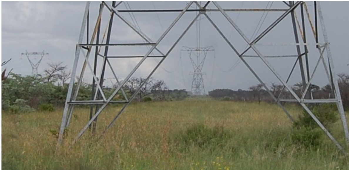
Figure 12: 132 kV (on the left) and 275 kV (on the middle) overhead power lines crossing the project site
