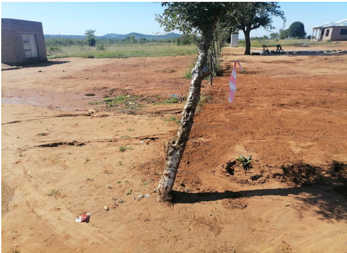
The danger tape indicate the peg where the pole will be planted
