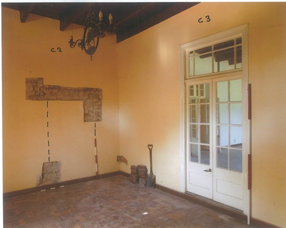
16. View in Room C2/3, where the earlier, blocked-up door is on the left (scales 2m, 1m, 50 cm) (look E).
