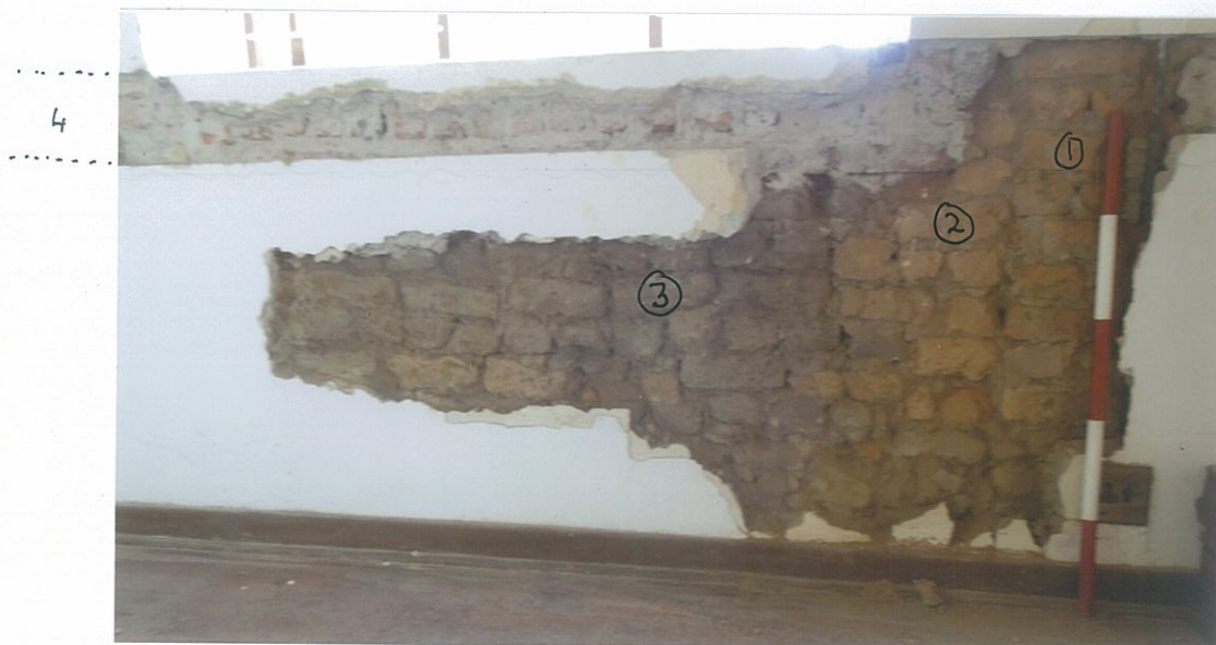
24. Close-up of wall F4 below the window-sill, of the different portions of brickwork (1 to 4) (scale 1m).
