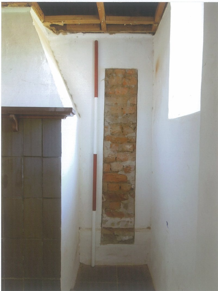
40. The band at the back shows homogeneous, well-fired orange brick with a stone plinth 35 cm high (scale 2m) (look S).
