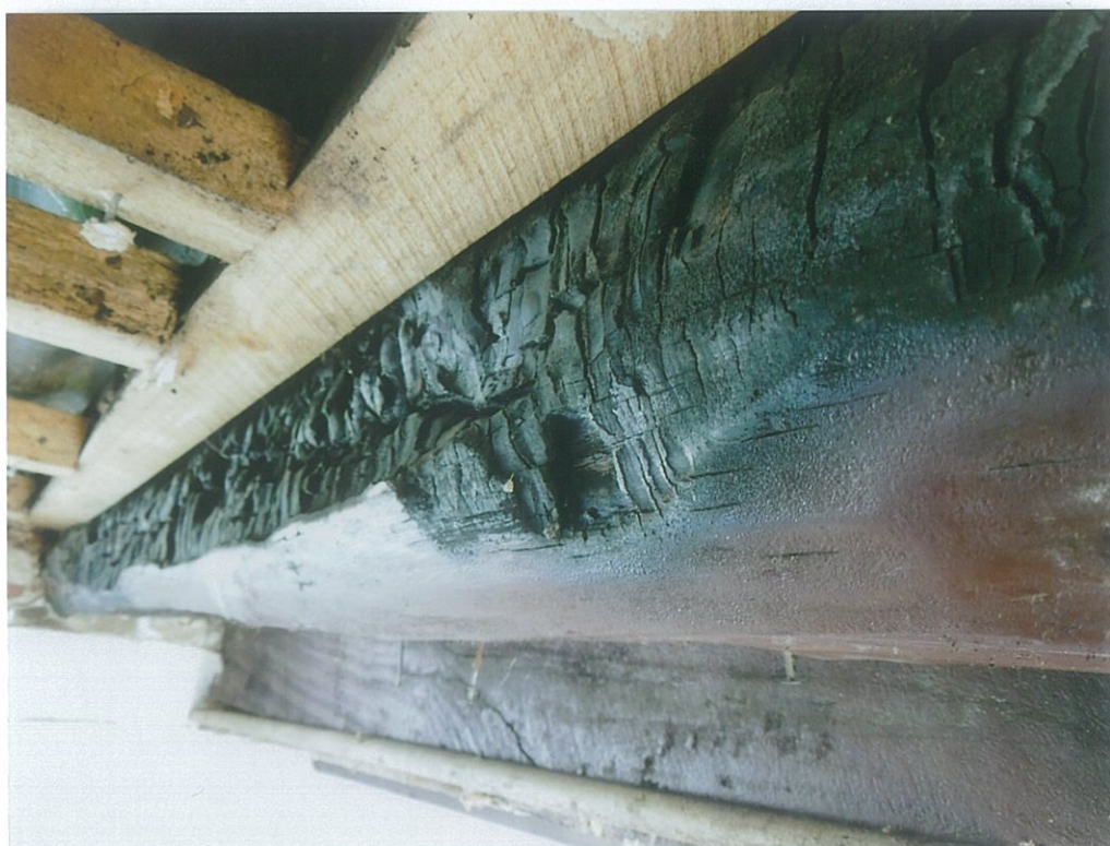
42. A view of the poplar beam heavily charred during a house-fire of the 19 th c (look W).
