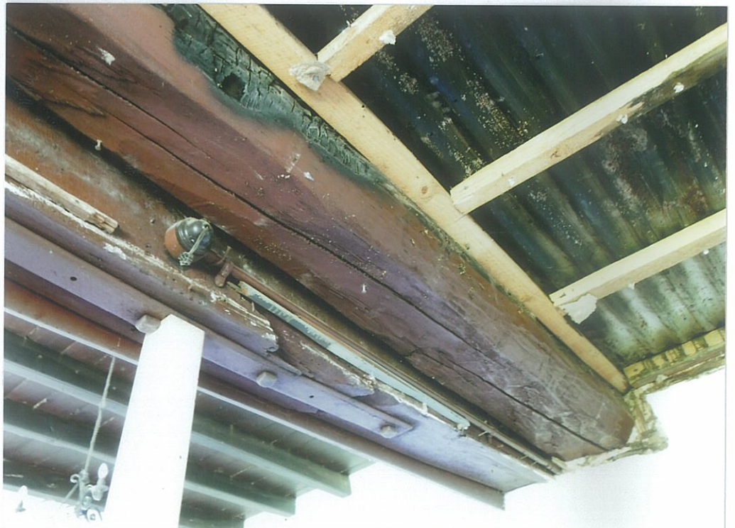
43. The other side of the carbonized poplar, circular beam where it resides next to the square hearth beam, mended with an iron strap to stabilize a crack in the wood (look E).
