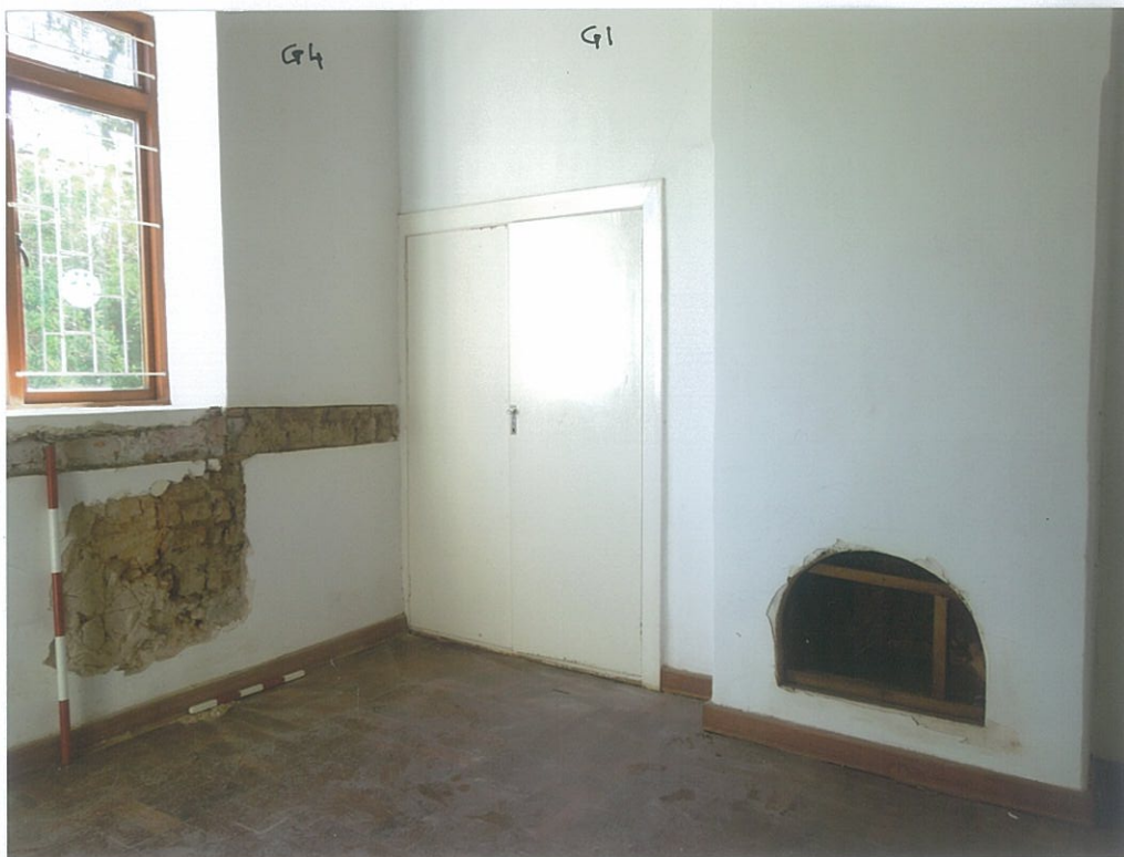
29. View of Room G4/1 of the plaster stripped, the blocked-up cupboard door and the opened-up grate of the late Victorian/Edwardian period (look NW) (scales 1m, 50 cm).
