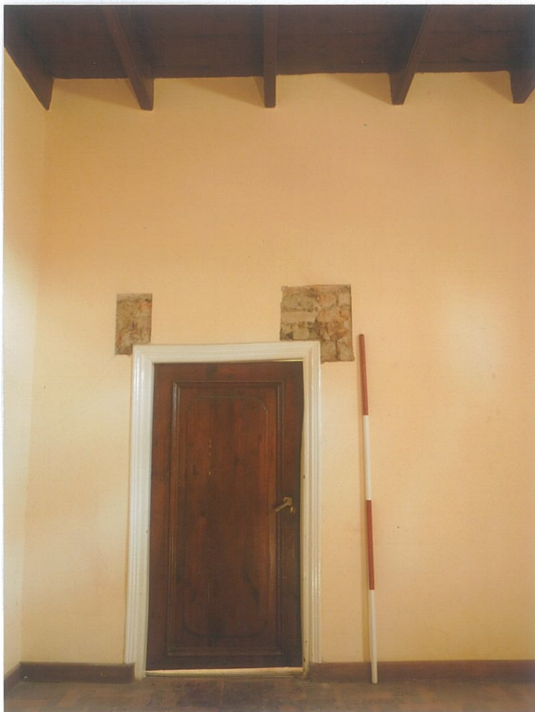
13. View towards wall C4 with the oldest door (mid-18 th ) with its surrounding architrave. Note its low position and the c.1880 beams overhead (scale 2m) (look W).
