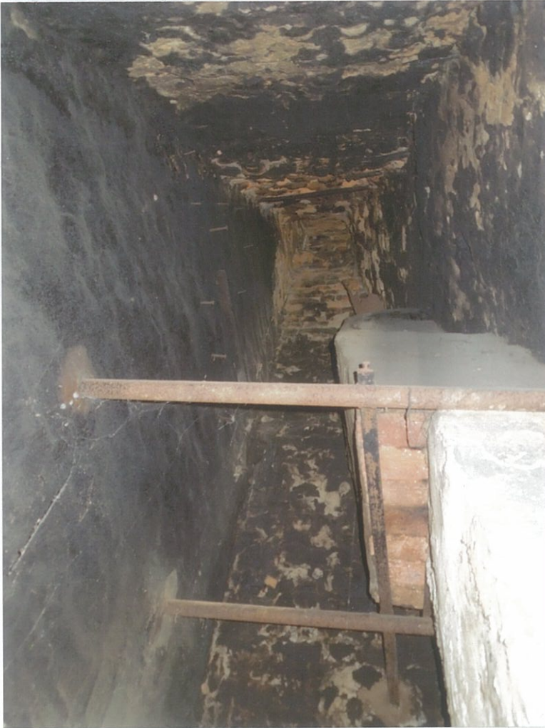
44. A view up the chimney, blackened by soot since 1800s. The structure on the right and the iron bars, date from the 1940s.
