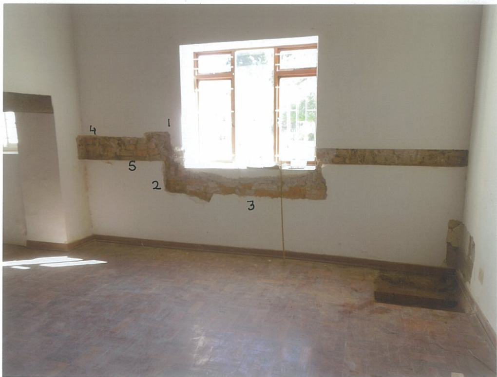
35. View within Kitchen I of Wall 4 where plaster was stripped in bands. The excavation is on the right (look W). The next photo (36) is of the left-hand corner.
