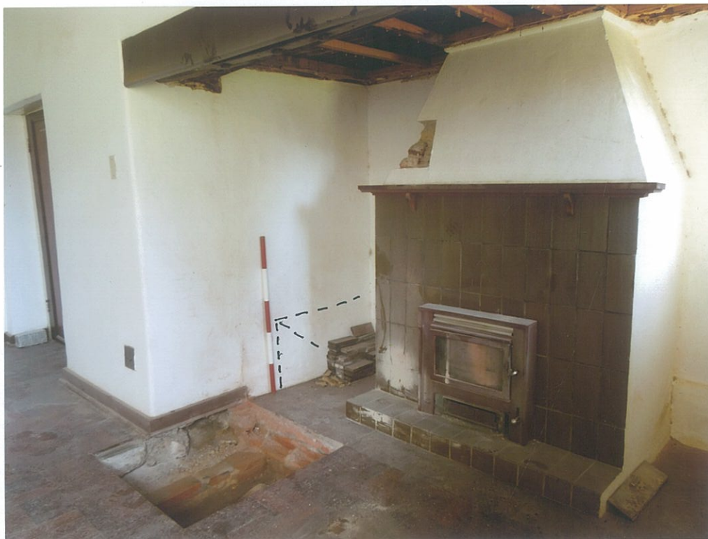
41. Another view of the c.1940 grate, hood and sloping chimney built-in position of the earlier hearth. The 1m scale stands about where the low original hearth would begin and raised about 45 cm (look SE).
