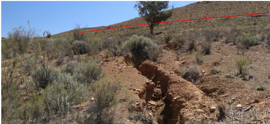
Figure 3: Storm water from the adjacent gravel road (red) does contribute to significant erosion on the site.
