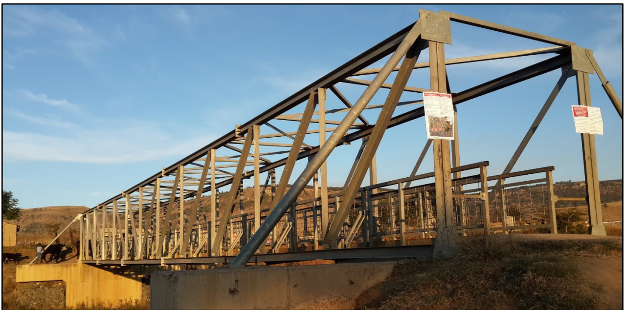
Plate 2: An example of a bridge along which pipeline will be tacked so as to avoid any construction within the watercourse
