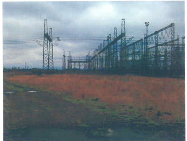
Looking West past Bighorn Substation
