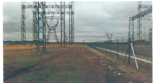
Looking North past Bighorn Substation
