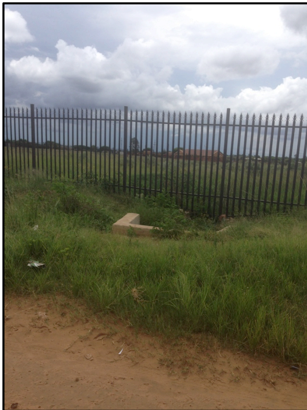
Photo 12: Small stormwater drain in area of 3,3km near east end of route
