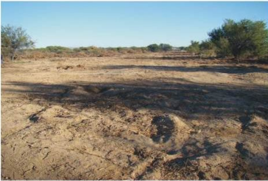
Figure 4. A 540 m long section between the R359 and the village (section A - B) has been stripped of vegetation to make way for the new road; looking southeast towards the village (above) and northwest towards the R359 (below).
