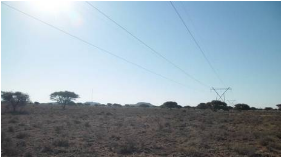
Figure 3: A section of the existing Kimberley DS Skietpan 132kV power line which the above alternatives are proposed to follow.
