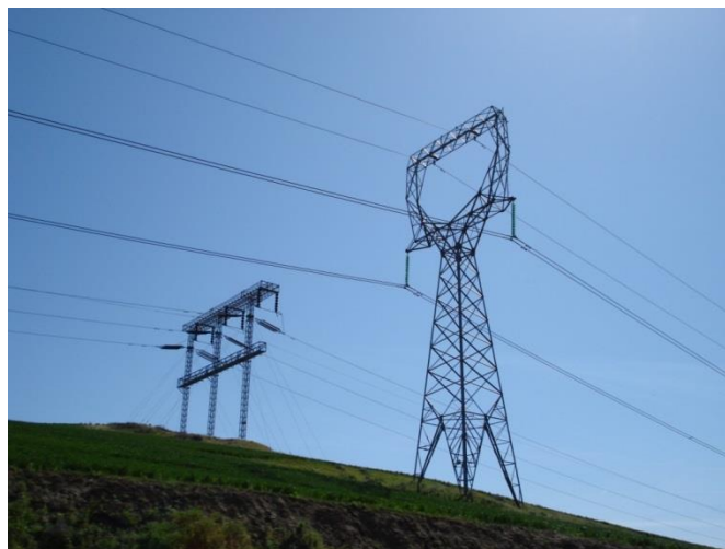
Figure 18: Example of a 143kV transmission line (Source: http://www.commonswikimedia.org (Accessed 9 July 2013))
