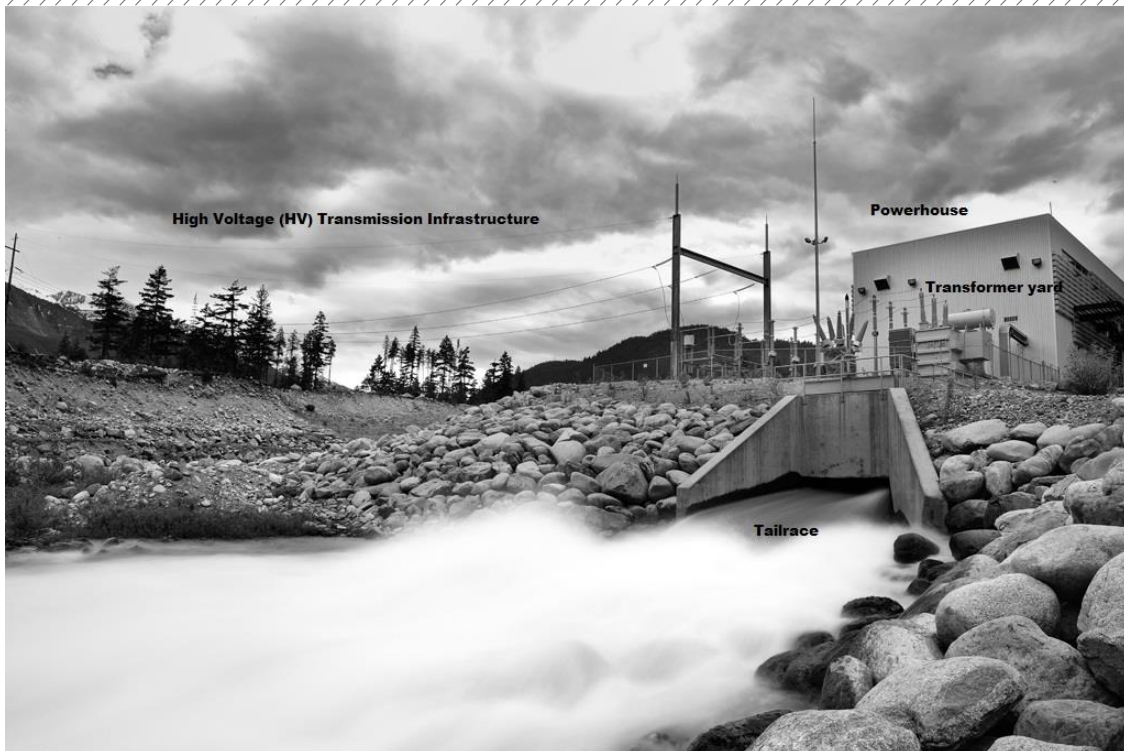
Figure 17: Example of a powerhouse and associated infrastructure. (source: http://www.photosensitive.com (Accessed: 28 June 2013)).
