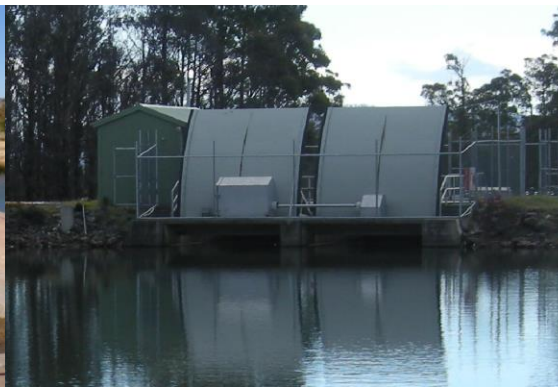
Figure 4 | Example of an intake structure with trashracks & gate. Note the proposed intake would not have a shed.
