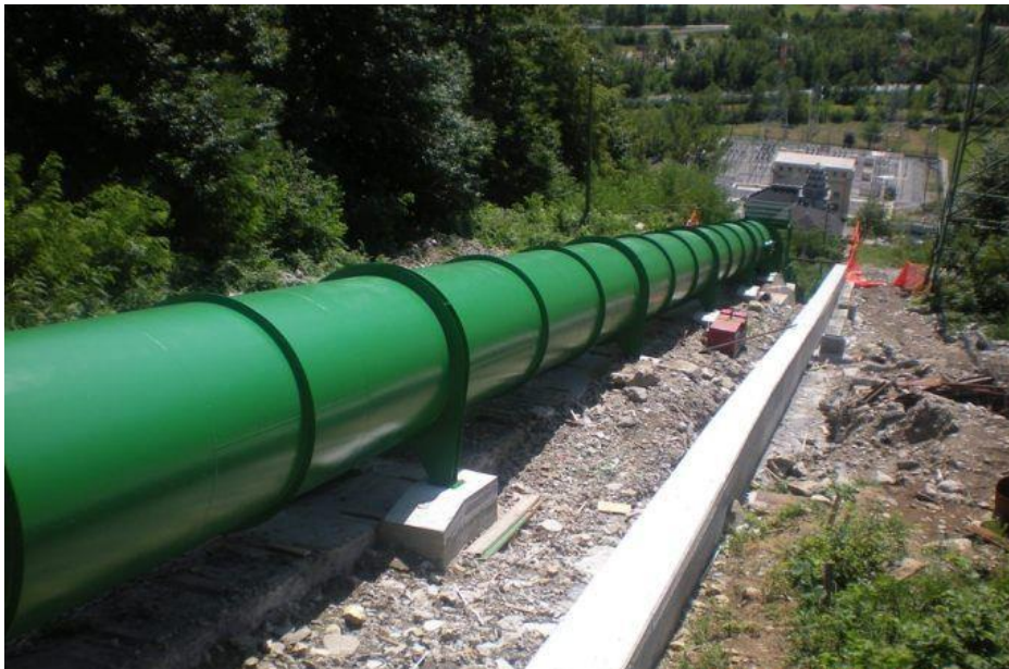
Figure 13 | Example of a penstock (source: energypedia.info (Accessed: 28 June 2013)).
