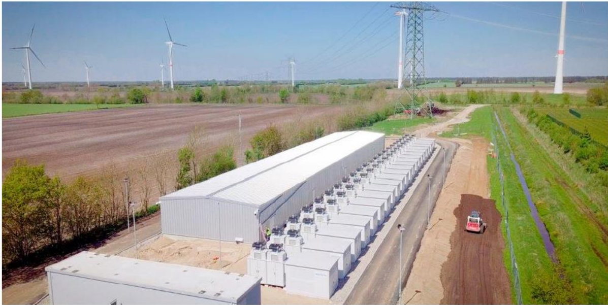
Figure 1.2: Typical Containerised Battery Energy Storage Facility
