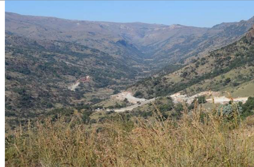
2-11b) Construction from BN to BS1/2 and to the Eastern Section of BS4
