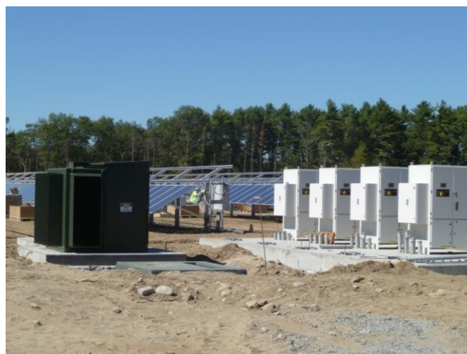
Figure 4: Inverter (Photo courtesy of BlueWave Capital SA)
