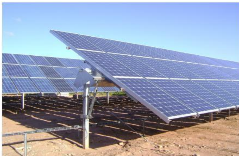
Figure 2.5: Solar arrays (static technology)
