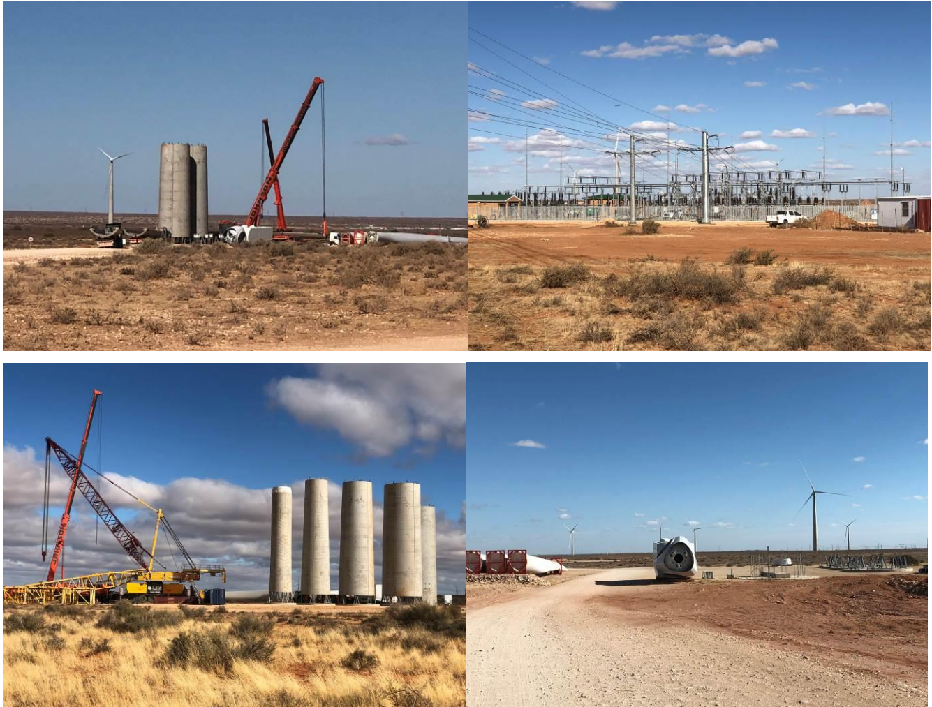
Figure 2-5: Photographs depicting the construction phase of a wind farm similar to Botterblom WEF.
